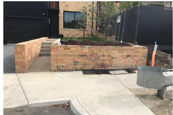
Wall after graffiti removal
